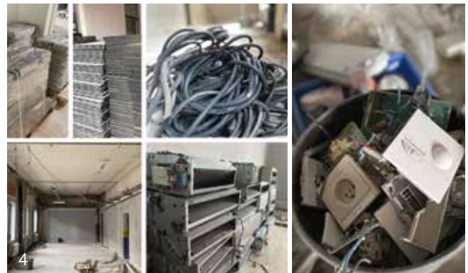
1) Circularium 2) Refurbishment of refectory for D’leteren Immo’s technical staff at the Kortenberg site 3) Färm supermarket at the Fort-Jaco site 4) Selective dismantling of the building on the Mobilis-project site
